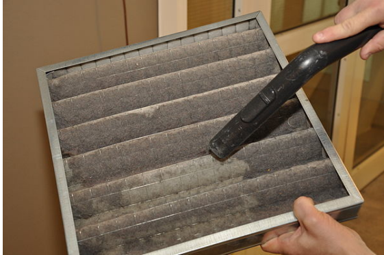
A common air filter, being cleaned with a vacuum cleaner
